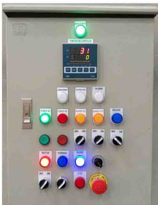
Digital Controller Panel burner
