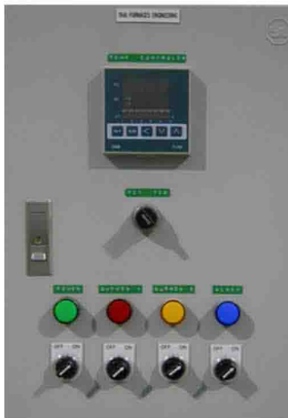
Digital Controller Panel burner
